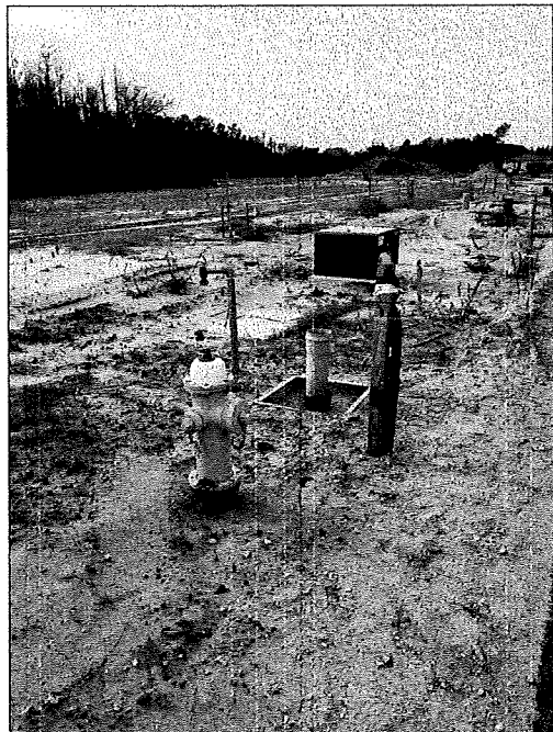
EXISTING PAD MOUNTED TRANSFORMER
